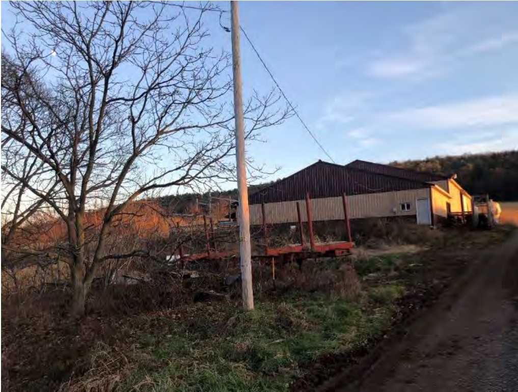
9 – North end of barn. Power line may need to be re-routed underground from pole to barn.
